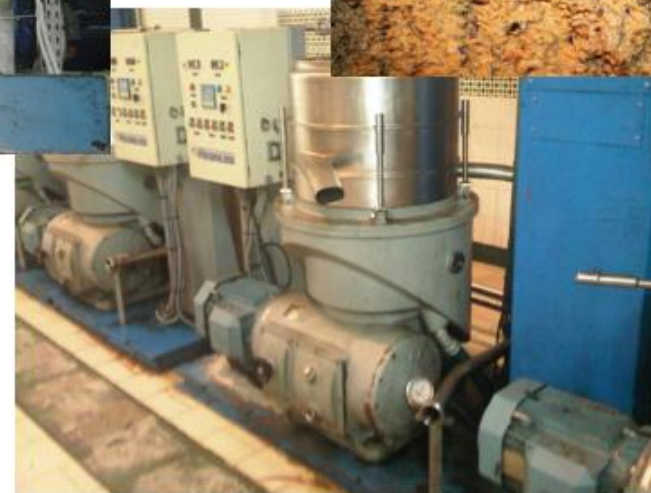
lubrification of malaxeurs / presses (leakages)
