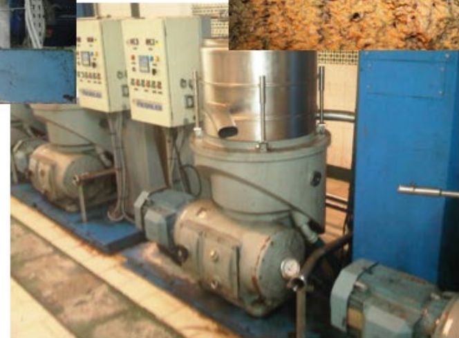
lubrification of malaxeurs /presses (leakages)
