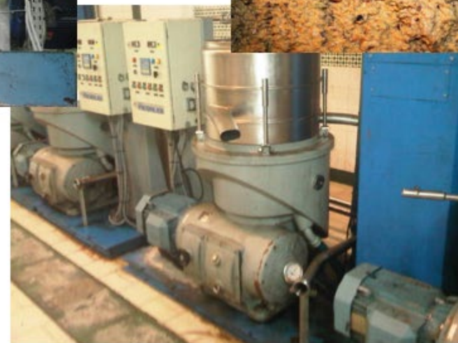
lubrification of malaxeurs /presses (leakages)
